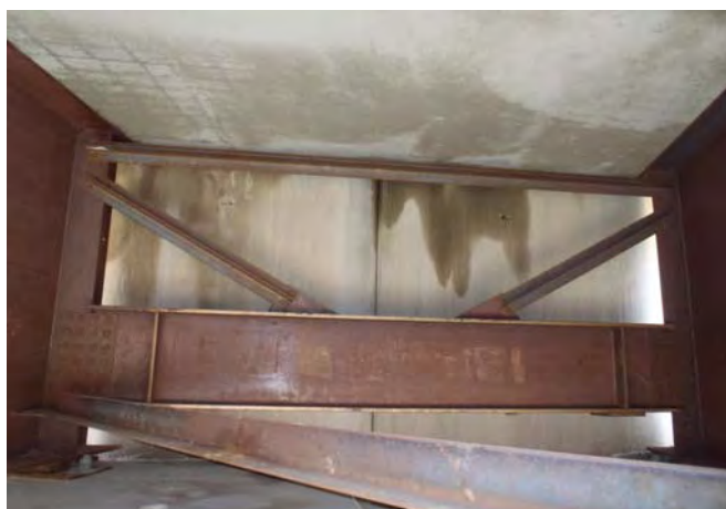
Figure 1-22: Camp end abutment, water staining of ballast wall.
