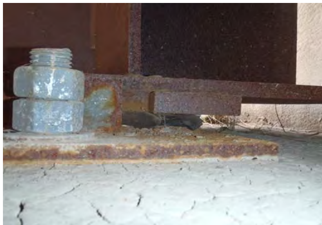
Figure 1-24: Typical deformation of camp end bearings.
