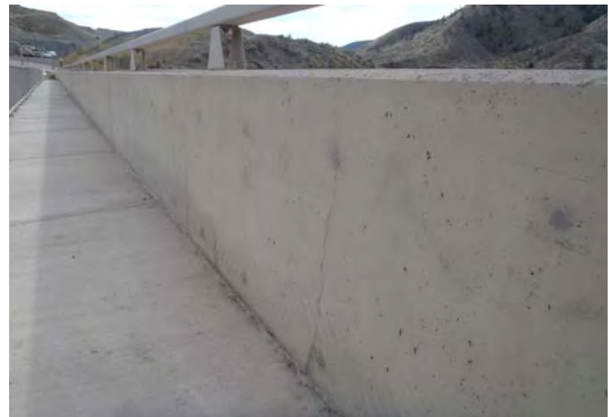
Figure 1-10: Typical parapet condition, note vertical crack.
