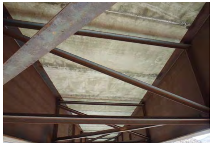
Figure 1-18: Typical sub deck and bracing condition, note staining around panel joints.
