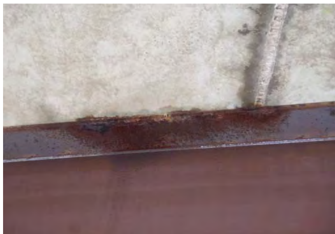
Figure 1-20: One location of steel flaking and pitting of top flange adjacent to grouted joint.
