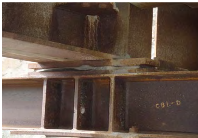
Figure 1-30: Typical bulging and deformation of pier 1 bearings, downstream shown.
