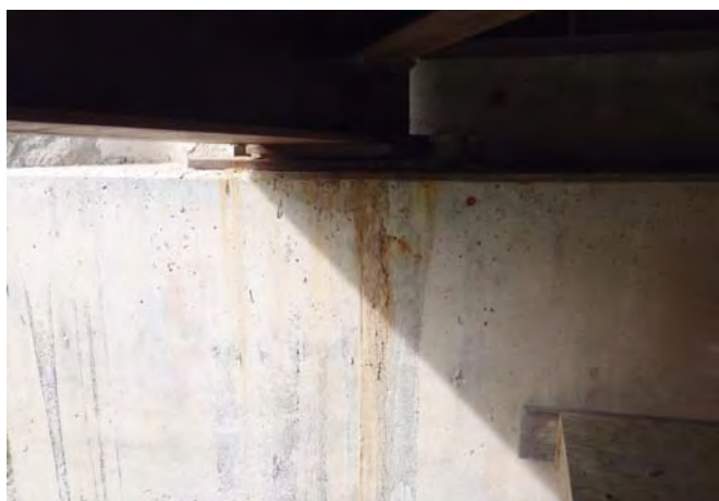
Figure 1-27: Woods end downstream bearing, corrosion staining on breastwall.
