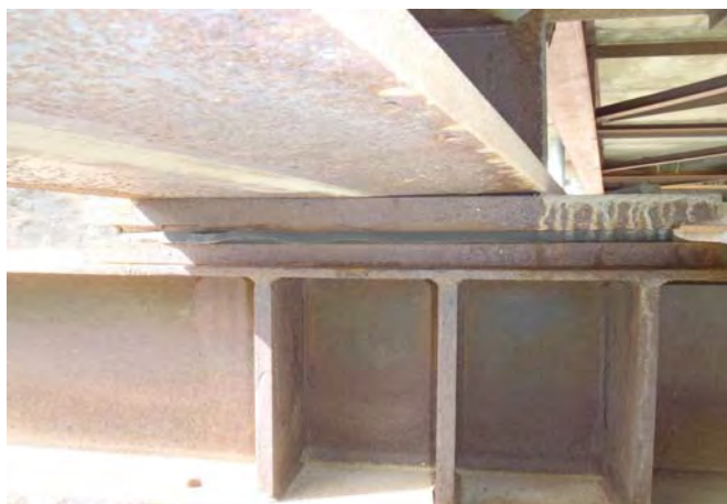
Figure 1-29: Typical bulging and deformation of pier 2 bearings, downstream shown.
