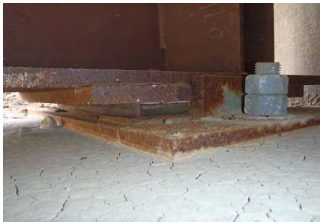
Figure 1-23: Camp end upstream bearing, note signs of water accumulation on bearing seat.
