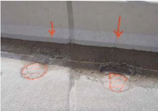
Figure 1-13: Marked delaminating grout pockets.
