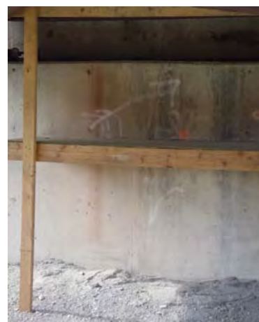
Figure 1-28: Woods end abutment, full height crack.
