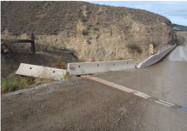
Figure 1-7: Camp end downstream barrier overturned.
