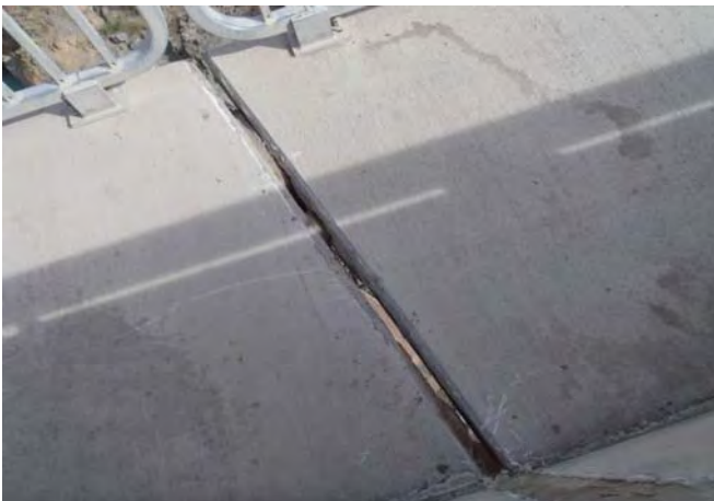
Figure 1-15: Pier 1 sidewalk joint, failed.
