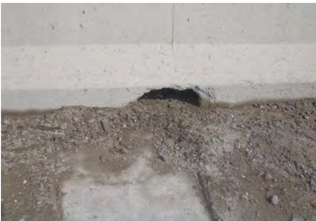
Figure 1-17: Woods end upstream drain blocked.
