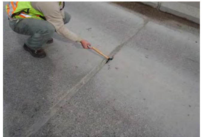
Figure 1-16: Pier 2 joint sealant debonded.
