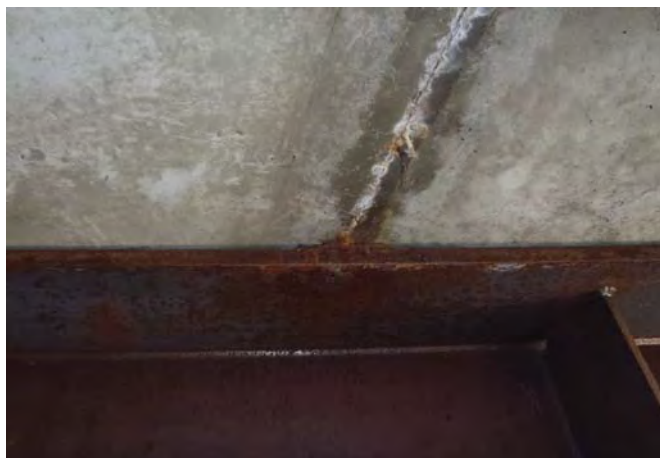
Figure 1-19: Typical corrosion of top flange at panel joint.
